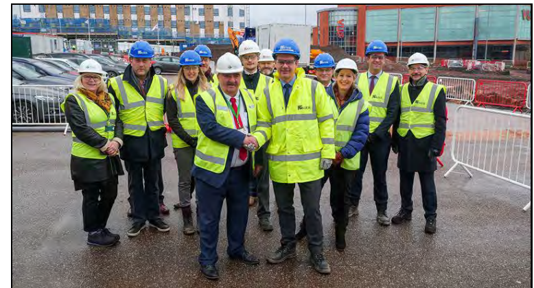
A formal ground breaking ceremony took place on 18 January. Pictured - Council Leader Peter Edwards and Kier's Managing Director, Anthony Irving, on site.
