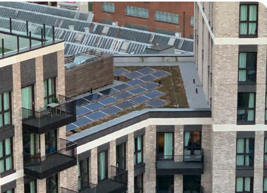
Photovoltaic array installed on higher density development, Wembley.
